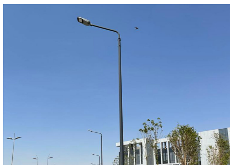
Milan luminaires in a commercial and leisure area of New Cairo City, Egypt
